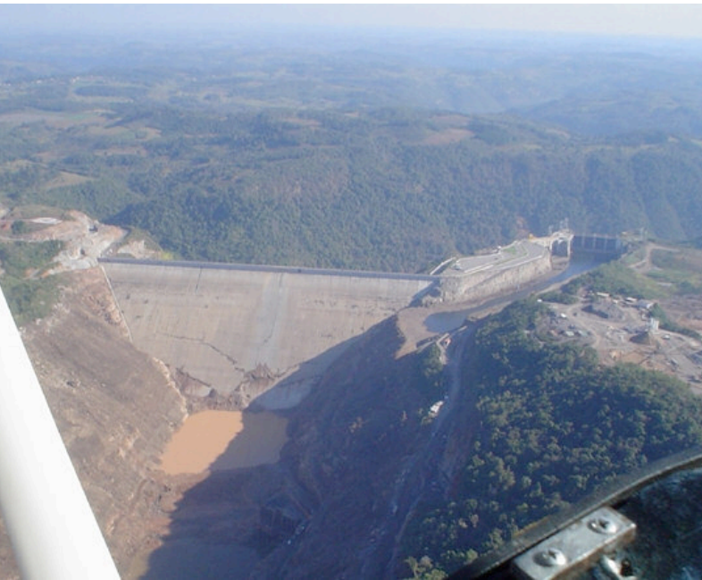
Damage to upstream side of Campos Novos Dam in Brazil after uncontrolled emptying of reservoir. This 880 MW completed project is seeking CDM validation.
